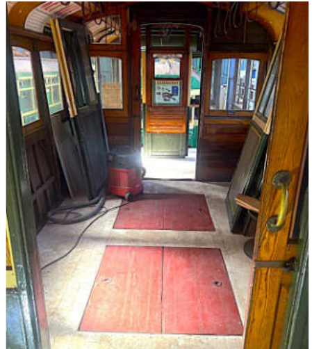
No.18 The floor has been replaced in the drop ends and saloon. Photo: Paul Mong
